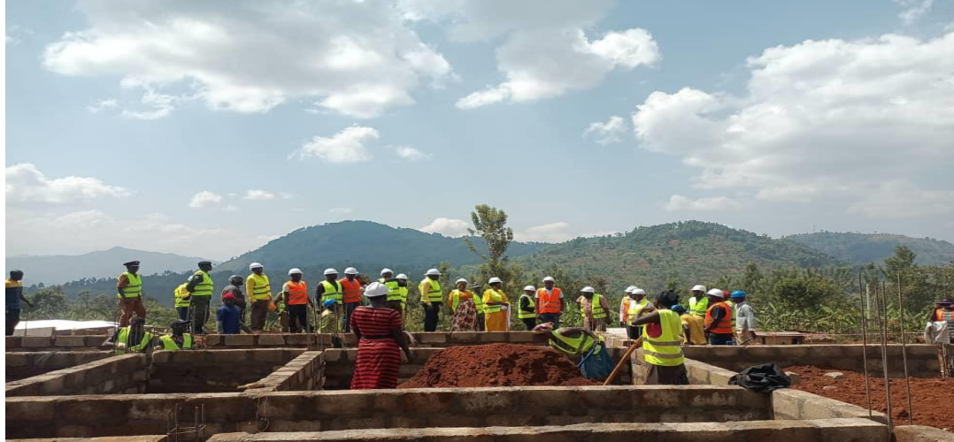
• Minister of Lands accompanied by the Minister of State for Karamojong inspecting the Construction of Nakatsi Seed Secondary School.
